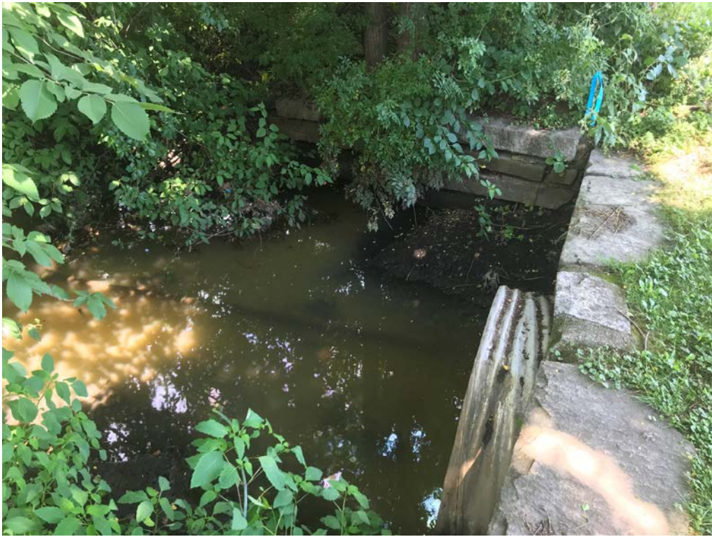
Photo 17: Aberjona River at culvert outlet near southeast corner of Castine Field.
