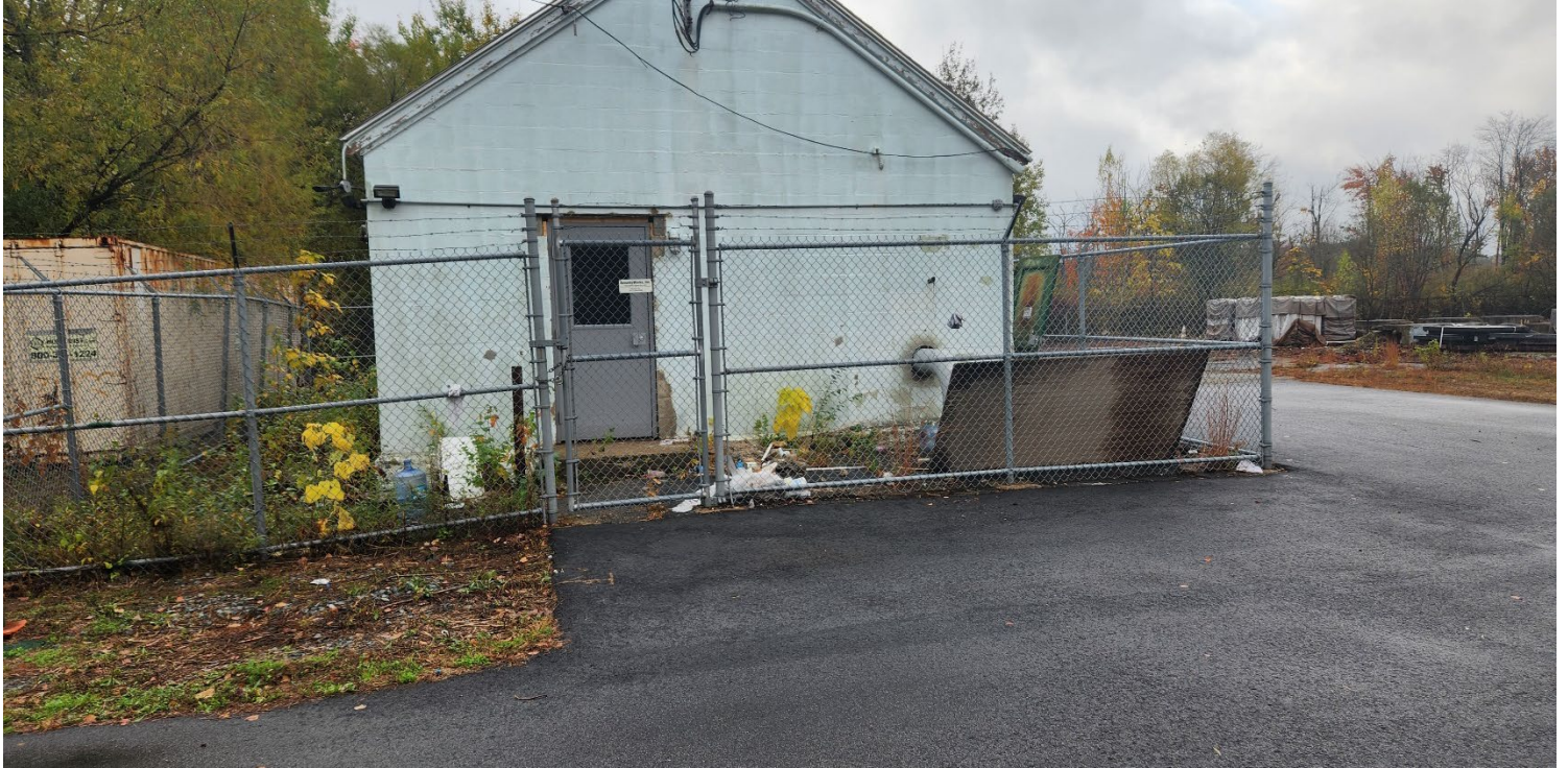
Photo #3: View of the front of the old pump building and internal security fence. The proposed liquid storage tank will be installed to the rear of the pump building (out of photo view), and the internal fence will be expanded to encompass the tank.
