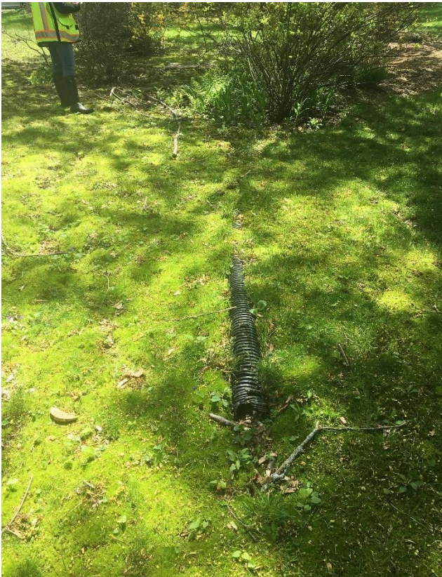
Photo 1. Corrugated tile drains observed in southwestern corner of site. View facing south; all photos taken on May 6, 2019.
