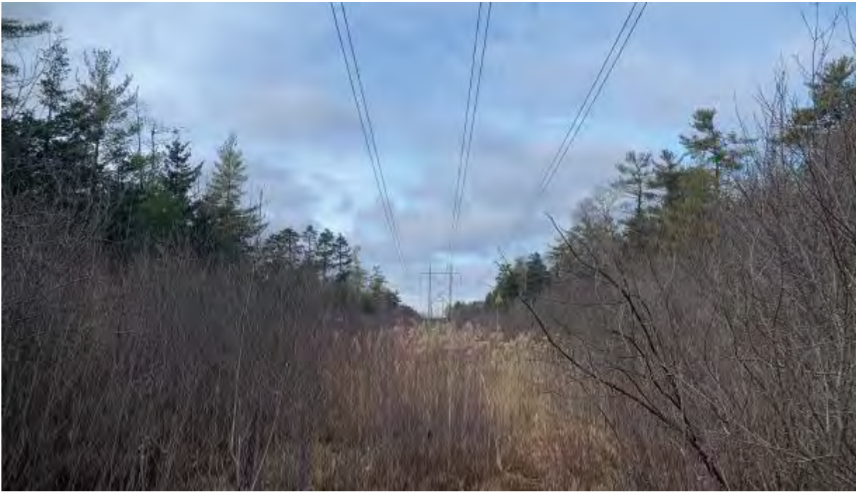
Photo 1: View of Structure 95 on the 339 Transmission Line ROW located within BVW. Facing northwest.
