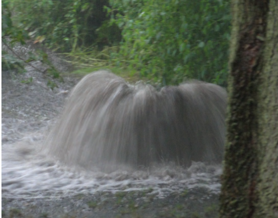
Figure 2-2. Photograph of Overtopping Manhole at 20 Bond Street
