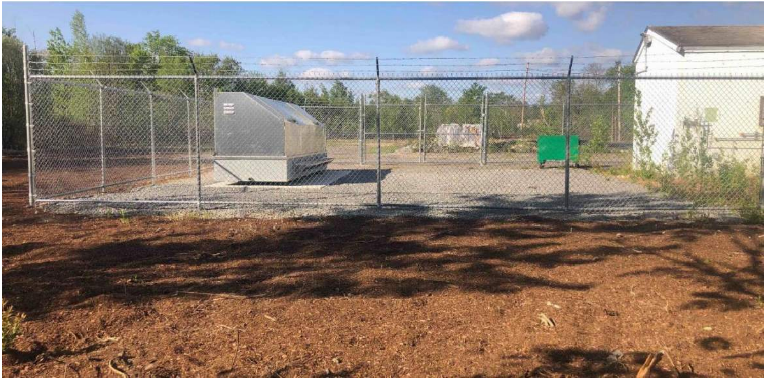
Photo #1: View of the gravel pad, storage tank, and existing building within the gas facility at 77 Walkers Brook Drive.. Existing garage foundation is visible through the fence in the background.
