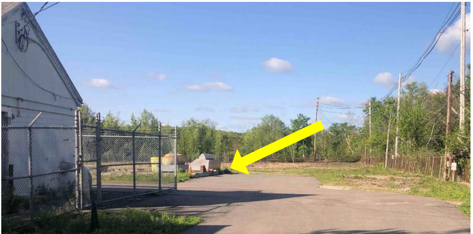
Photo #2: View of the existing foundation, as it is being used for temporary storage of equipment. Facing southwest.
