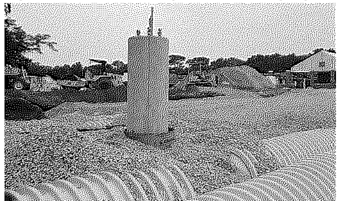
Figure 13 - Chamber bed placed around light post.
