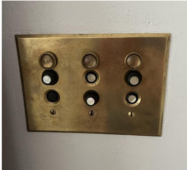
Original push button light switches in front entry.
