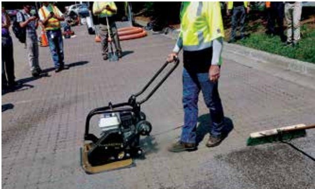
Figure 25. No matter the equipment used, after removing sediment soiled aggregate, clean aggregate is placed in the joints, the surfaced cleaned and compacted.
