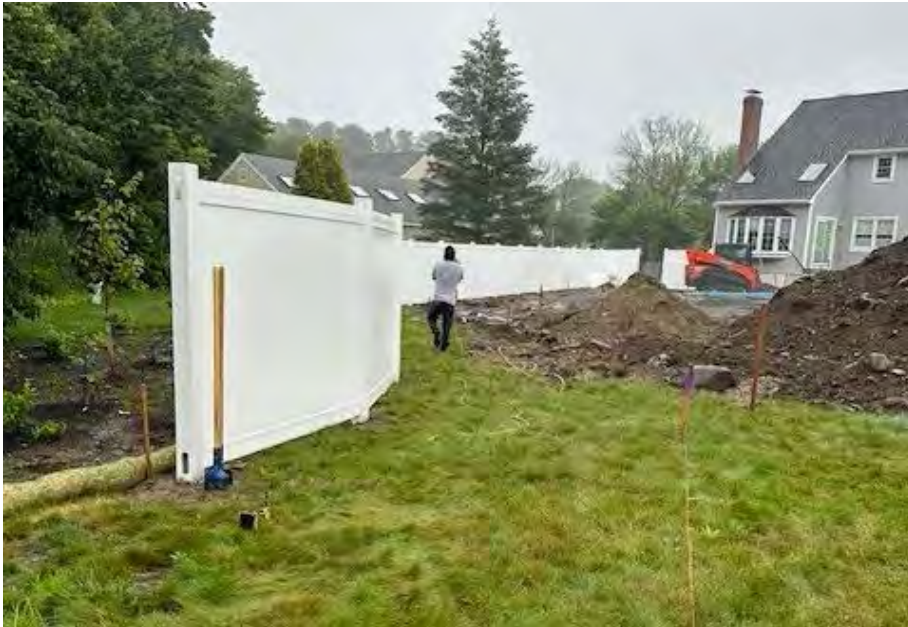
Photo #7: General view of fence installation during construction. Photo taken by landscape field crew.
