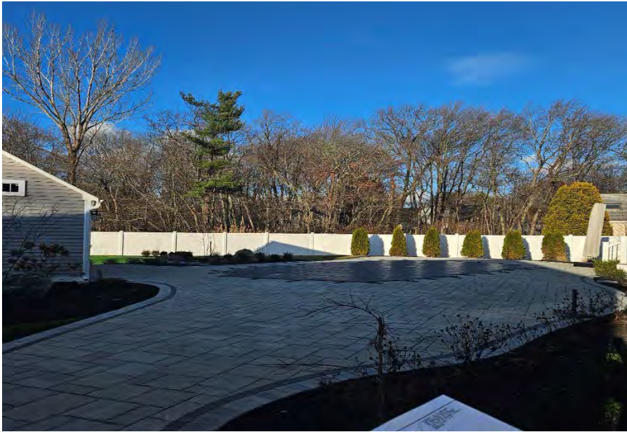
Photo #11: General view within new fence post-construction. Photo taken on November 28, 2023, by Hancock Associates staff scientist.
