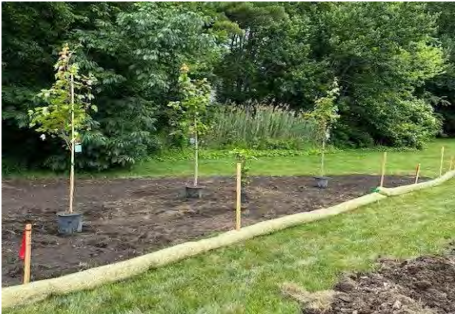
Photo #8: General view of plant installation during construction showing trees and proper erosion control measures. Photo taken by landscape field crew.
