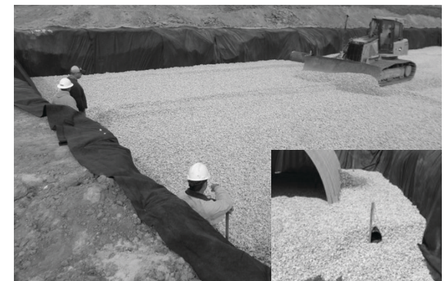
Place clean, crushed, angular stone foundation 6" (150 mm) min. Compact to achieve a flat surface.
